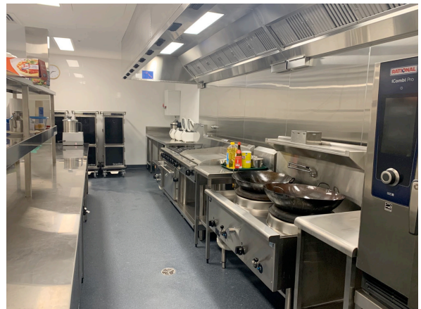
Culturally specific commercial kitchen
